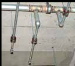
Fire Sprinkler Systems
